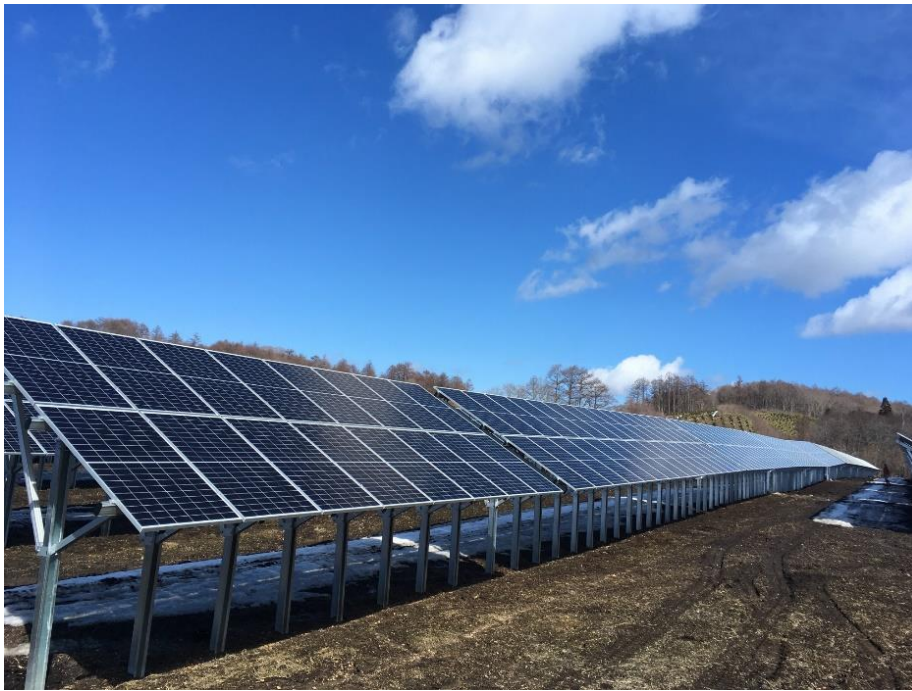
The Solar Power Plant in Shikabe
