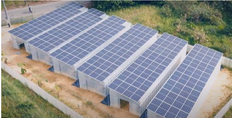
(“Sustaina-Cacao” Solar Power Plant)
